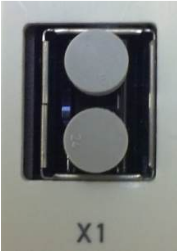
Figure: Blind plugs in unused sockets
